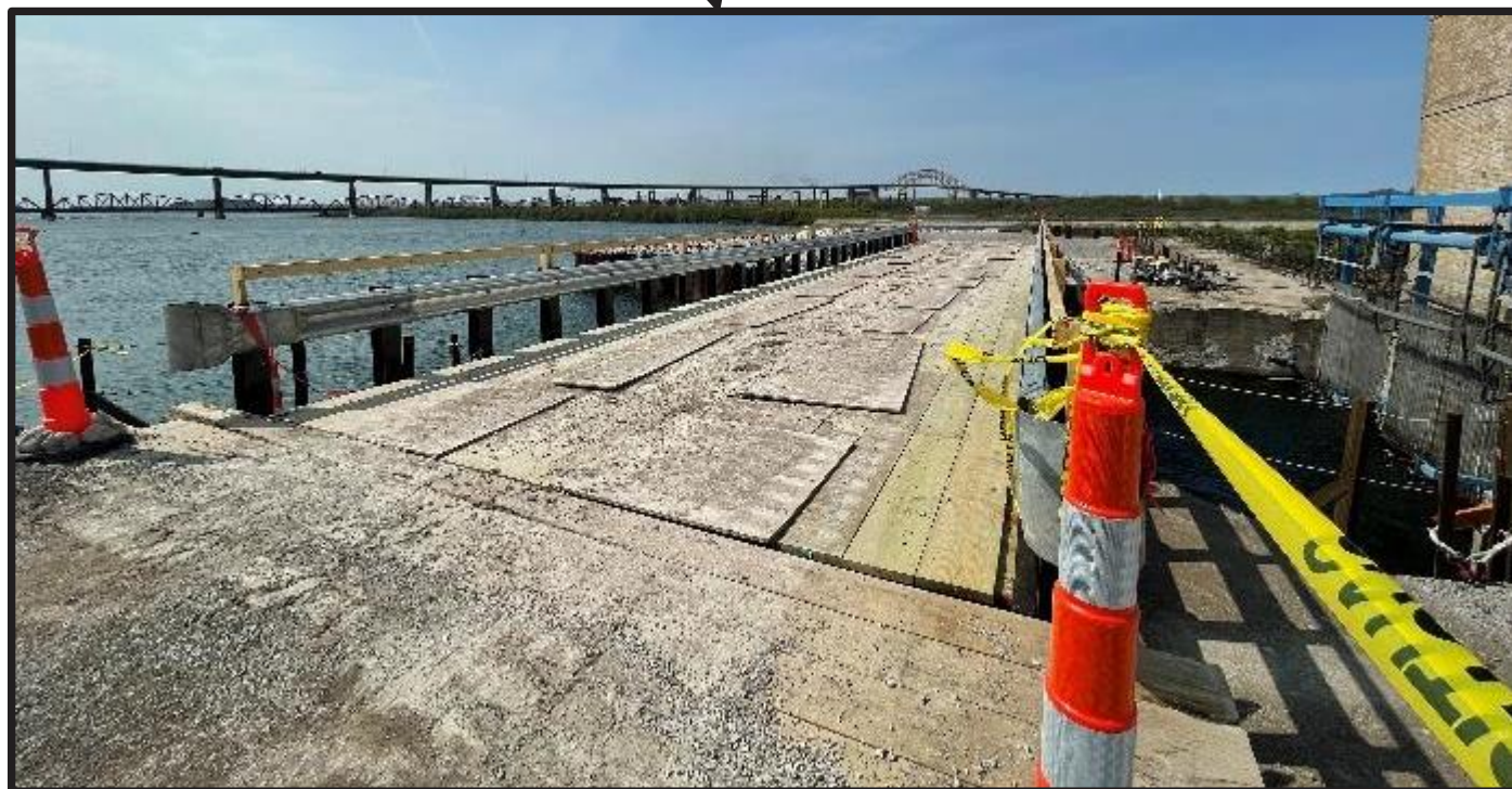
Prefabricated steel bridge installed west of Unit 10, providing haul route access to the Center Dike fill area
