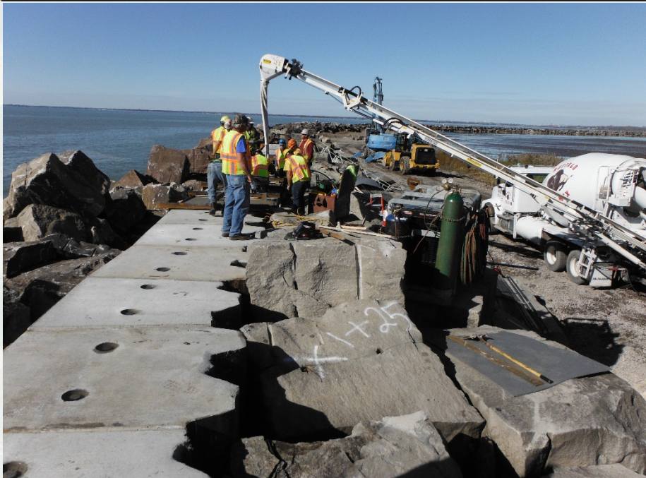
Looking down dike wall, showing finished concrete blocks and new blocks being poured.
