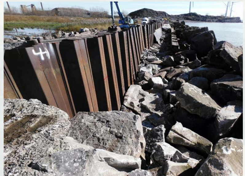
Looking toward shore, showing old armor removed and underlayer installed. Further out you can see that the underlayer has been grouted.
